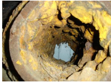
Tuberculated Unlined Cast Iron
