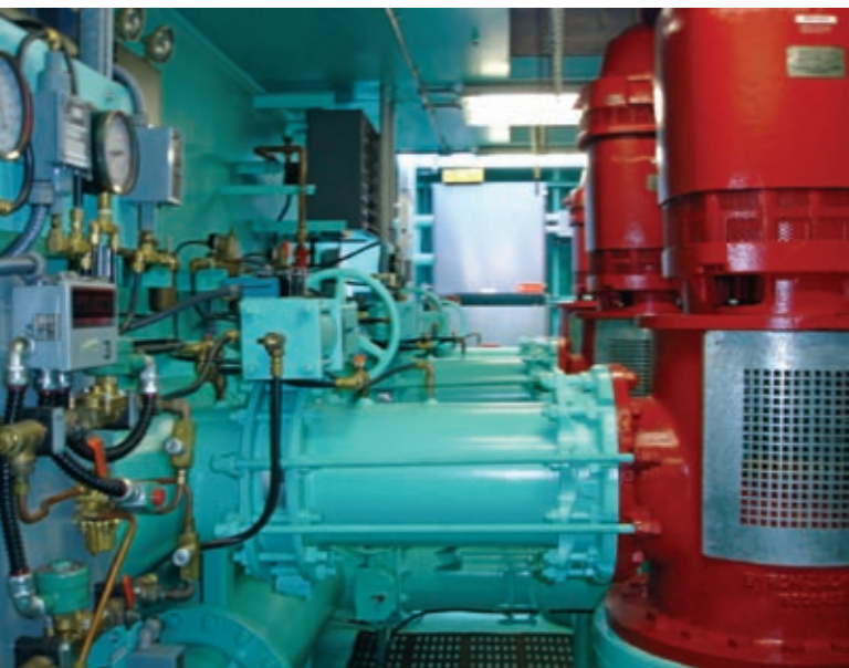
Setian Lane High Service Booster pump station.
